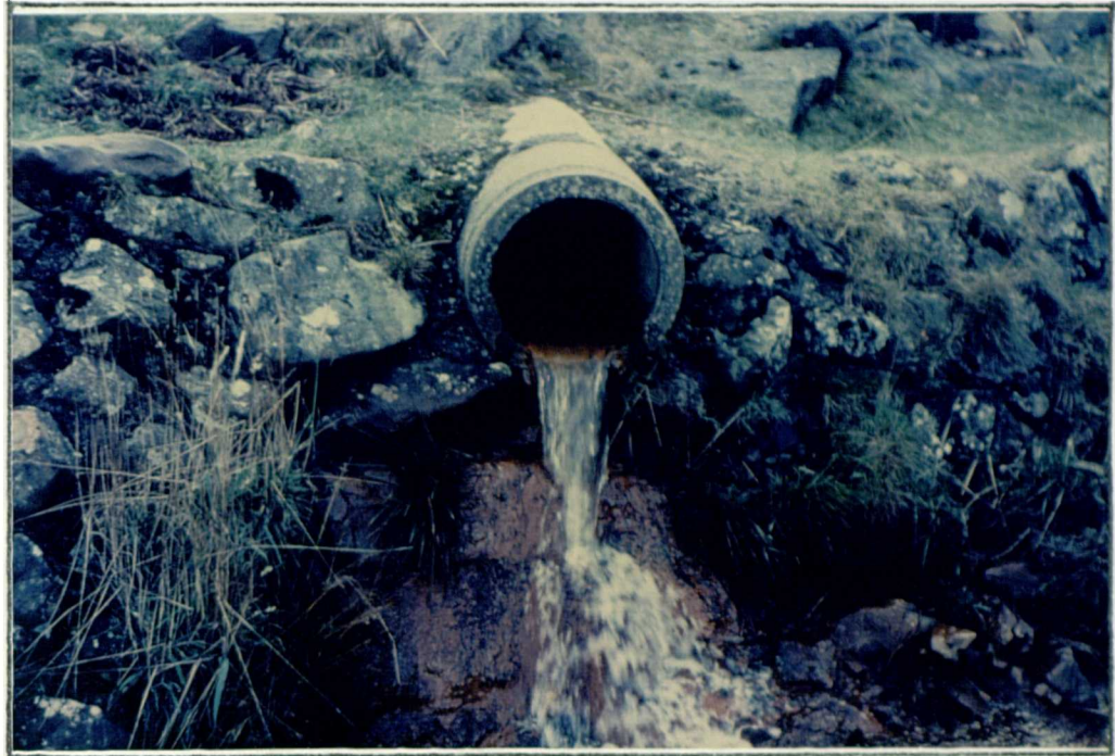
Plate 3:11 Llyn Cowlyd site 4 : This culvert conveyed water from the ditch shown in Plate 3:10 to a small river.
