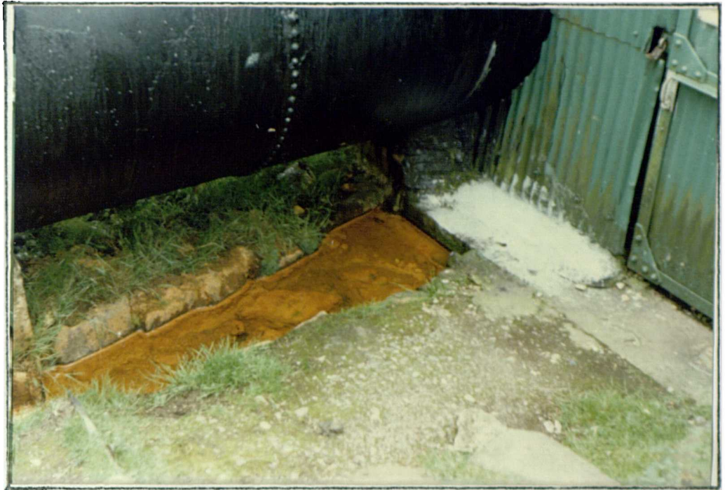
Plate 3:5 Llyn Coedty site 2 : Water entered the ditch via a culvert. The culvert is not evident in the photograph but runs diagonally from the bottom right to the centre.
