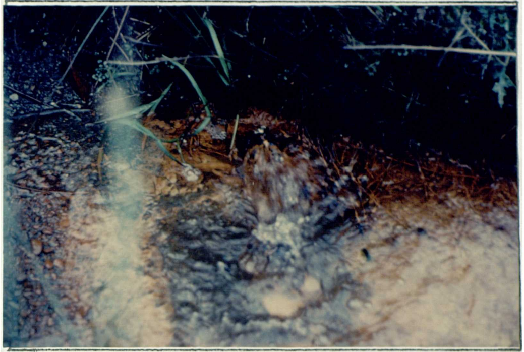
Plate 3:9 Llyn Cowlyd site 1 : Water bubbling to the surface at the head of an open ditch.
