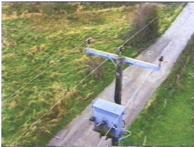
Figure 1.1: Example Support Pole showing 3-phase Conductors on Pin Insulators and a Pole-mounted Transformer.
