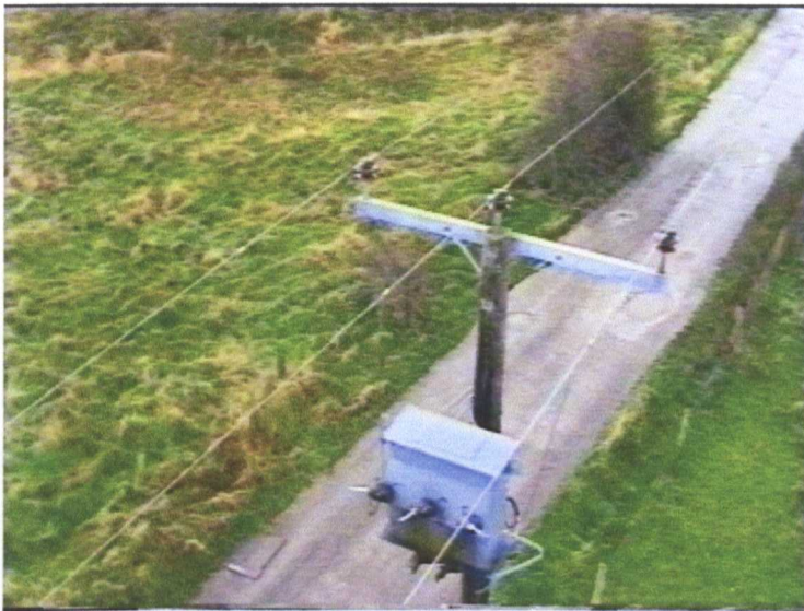
Figure 1.1: Example Support Pole showing 3-phase Conductors on Pin Insulators and a Pole-mounted Transformer.
