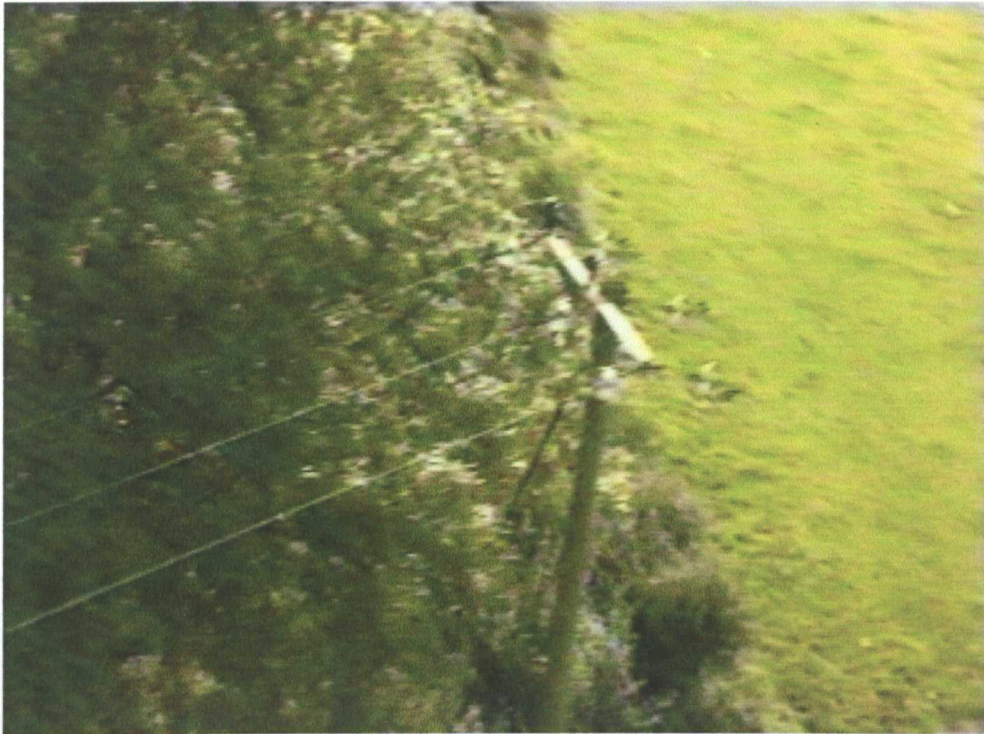
Figure 2.1: Tree Encroaching on a Power Line.
