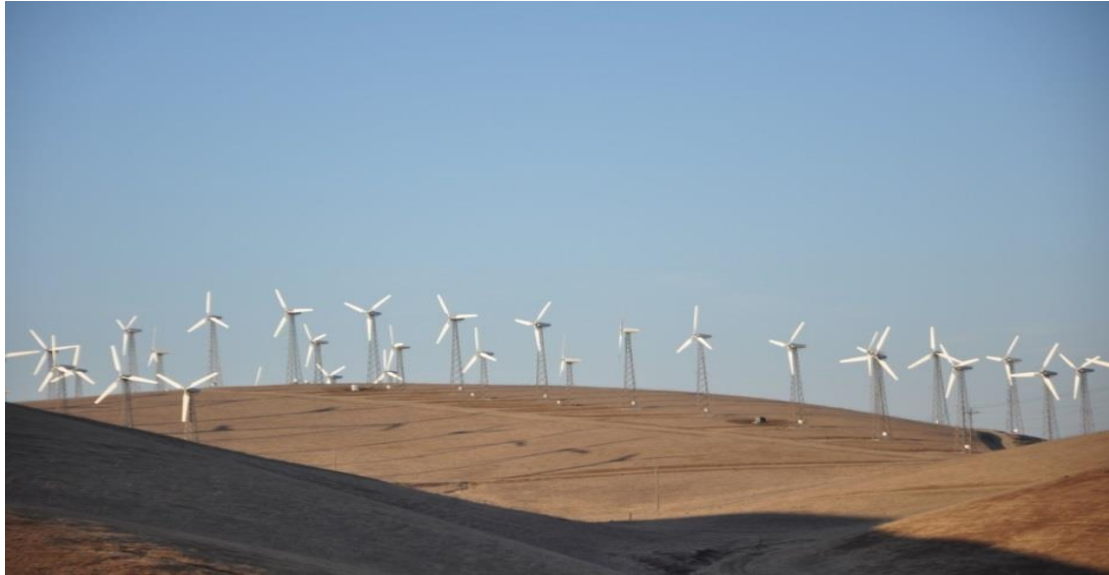
Figure 15: Altamont Pass Wind Energy Development
