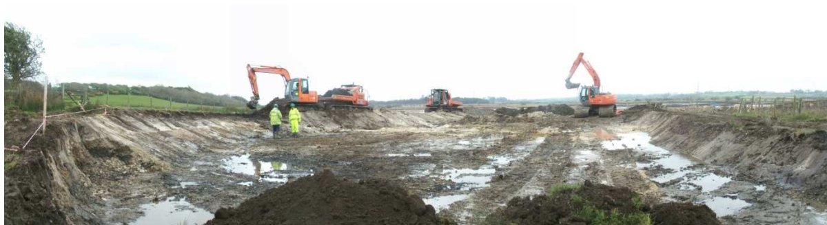
Figure 4.6 – View from the inlet zone during construction phase with civil engineering contractors at Cae Gwyn FWS CW.
