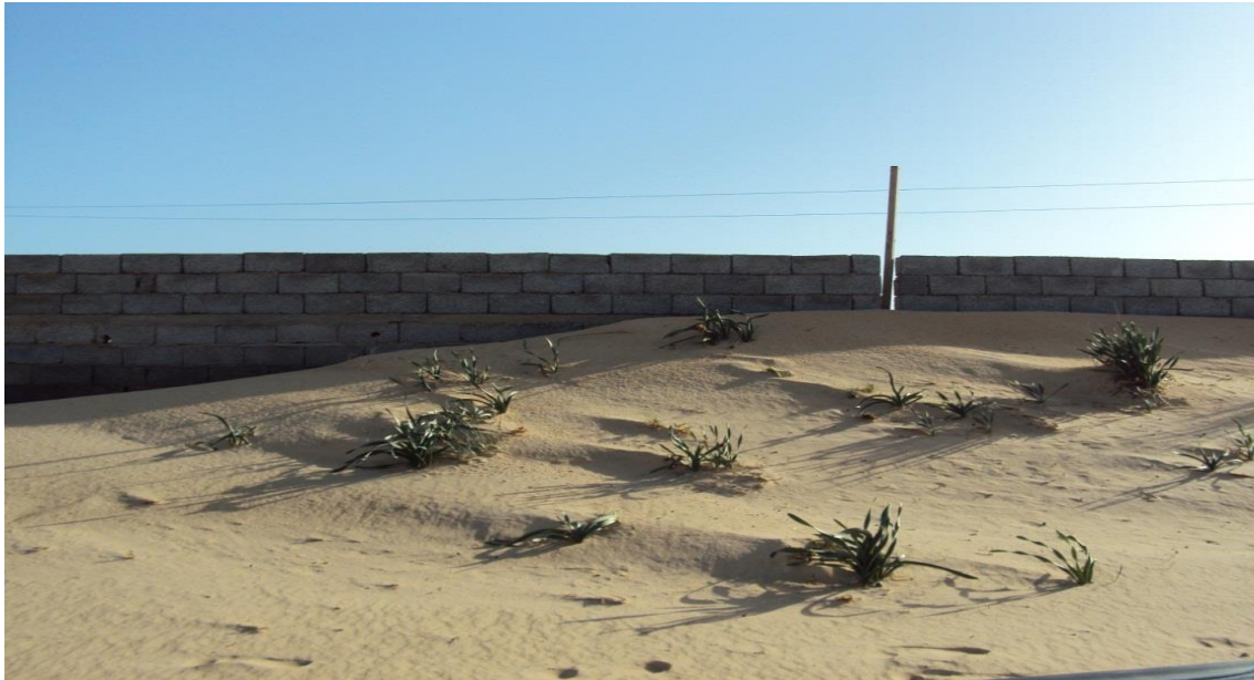
Figure 4.2: A wall built to prevent sand dunes encroaching, Alkarawh village, Al-Garabulli district (Source: Picture taken on 05.01.2013 by the researcher).
