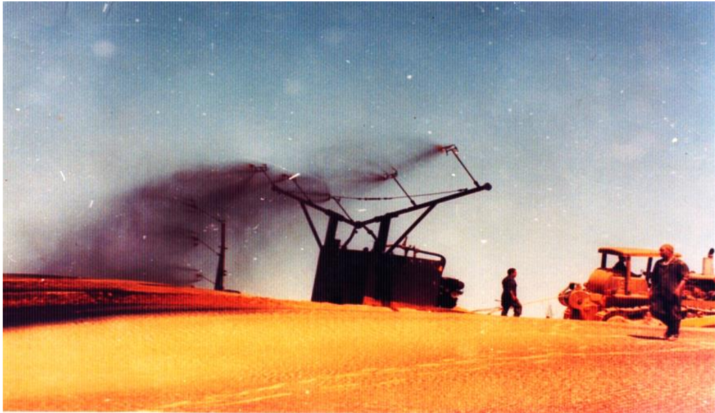
Figure 2.18: Sand dunes stabilization by using crude oil: The process of sand dunes stabilization by bitumen spray by a bulldozer which pulled the tank over the dunes ,in Al Atayah village in Algarabulli district in 1971 (Khatabi, 1981).
