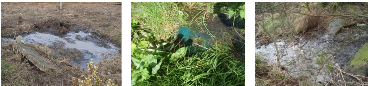
Figure 2.14: Indicative signs of ST failure: Left: showing broken tank lid exposing the effluent to the environment. Middle: showing effluent discharge (blue colouration) leaking on to the surface. Right: showing effluent flooded on to the surface above the tank lid. Photos were taken during PhD field work.
