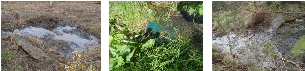
Figure 2.14: Indicative signs of ST failure: Left: showing broken tank lid exposing the effluent to the environment. Middle: showing effluent discharge (blue colouration) leaking on to the surface. Right: showing effluent flooded on to the surface above the tank lid. Photos were taken during PhD field work.
