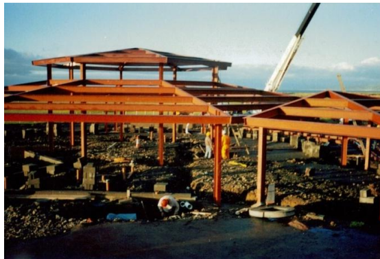
Photo 3.52. Structural steel work for Llyn y Gele Clubhouse. Reproduced by kind permission of the Williams family.
