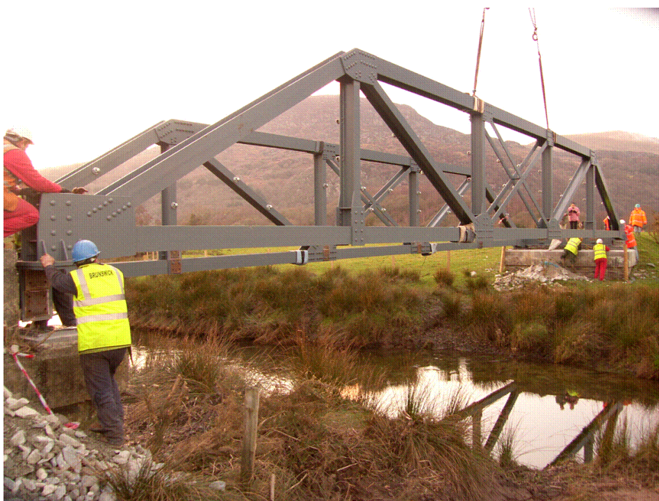
Photo 3.56. Installation of Dylif Bridge March 2007. From the Brunswick Ironworks Archive reproduced with their kind permission.
