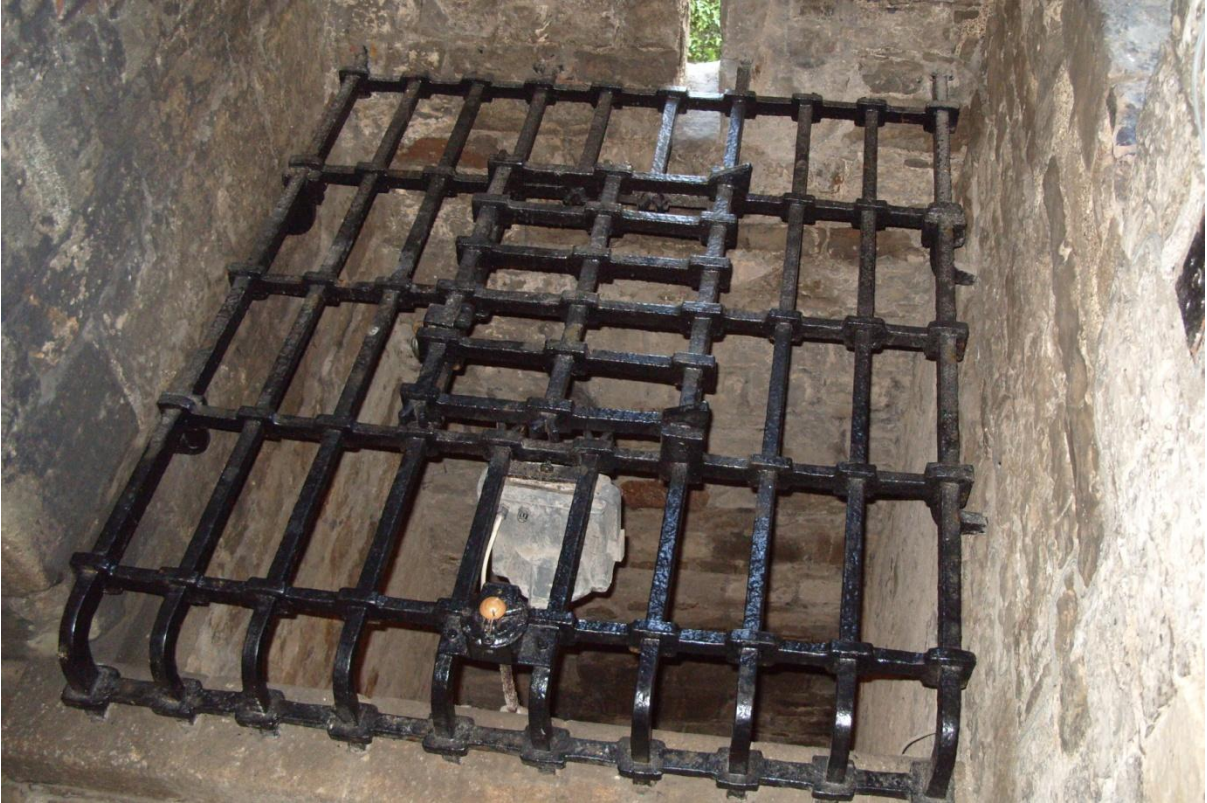
6.3. The well cover located within the Well Tower designed and installed by DJ Williams. Photographed by Pam Smith 2011.
