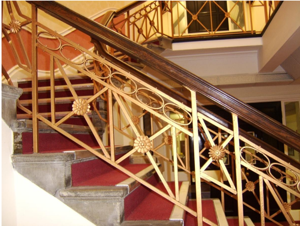
Photo 3.15. Staircase railings designed by DJ Williams for County Offices Caernarfon 1931. Photographed by Pam Smith with kind permission from Gwynedd County Council 2006.
