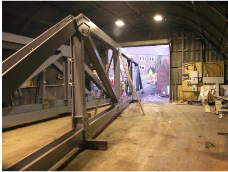
Photo 3.55. Under construction Brunswick Ironworks 2008 the Pont Croesor Bridge. Reproduced from the Brunswick Archive with their permission.
