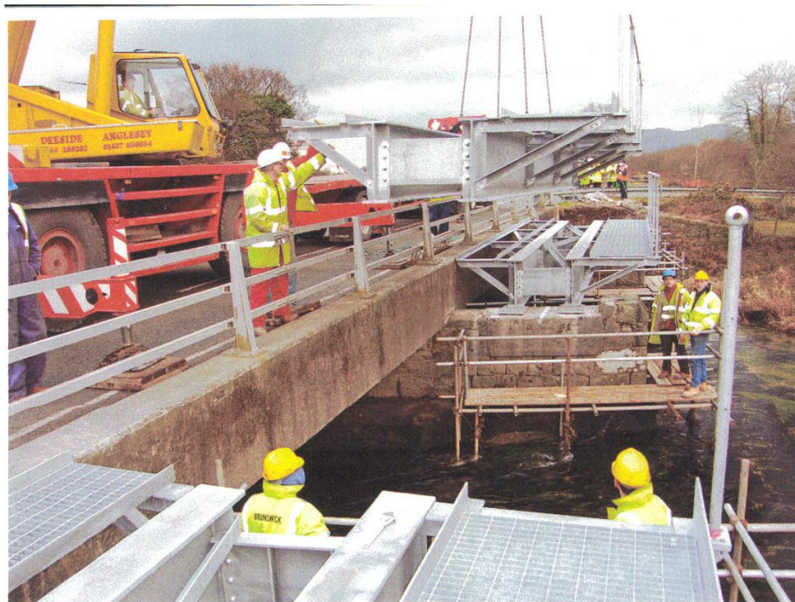
Photo 3.54. Nantmor Bridge installation October 2006. Reproduced from the Brunswick Ironworks archive reproduced with their kind permission.
