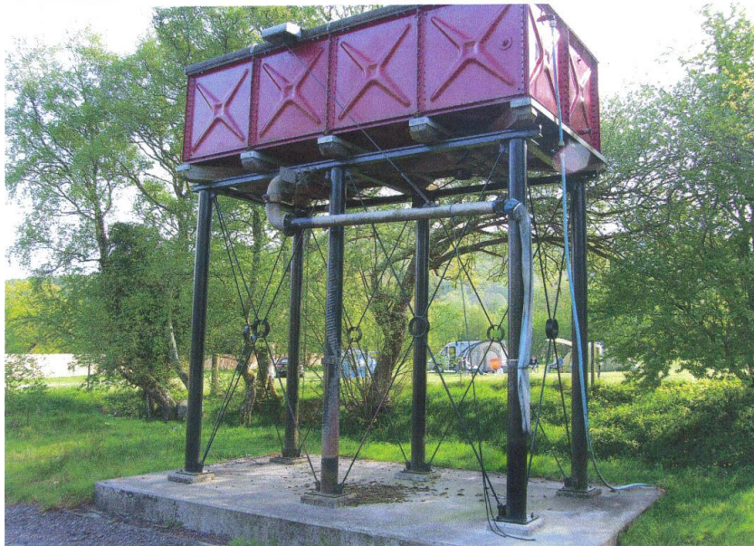
Photo 3.59. Water tank steel frame constructed for the Welsh Highland Railway Dinas Station Caernarfon. Photographed by Pam Smith. 2009
