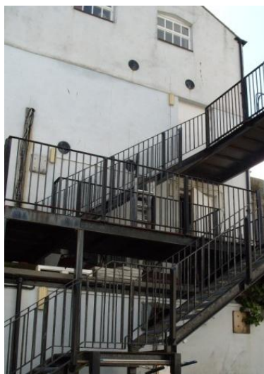
Photo 3.29. Metal fire escape Corn Mill Palace Street. Photographed by Pam Smith 2009 reproduced with the kind permission of the owners of the building.
