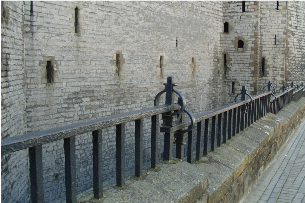
6.1. The railings designed and installed by DJ Williams for the 1911 Investiture of the Prince of Wales. Photographed by Pam Smith 2011.
