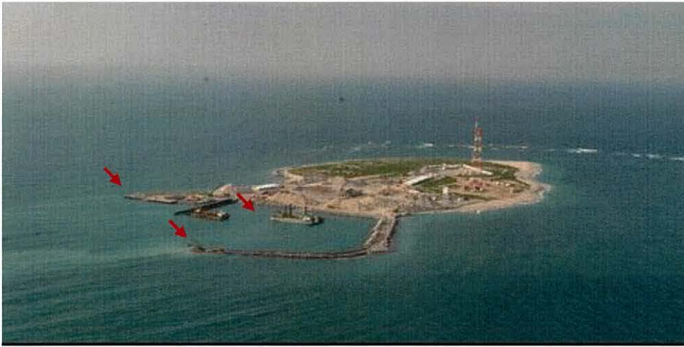
Figure 6.4.9. The new marina during construction showing dredging activities with red arrows were causing high turbidity at Umm AlMaradim in December 2005.
